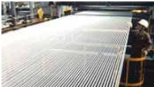
In 1970, installed German-made equipment for producing a 3.2-meter wide steel cord conveyor belt at the Hiratsuka Factory.
